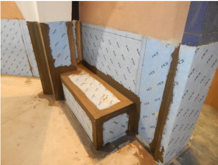
The raw form of the heated benches consists of PCI PowerBoard HR foam boards waterproofed with PCI Pecilastic W. ( Link to high-resolution photo, ©PCI Augsburg GmbH)
