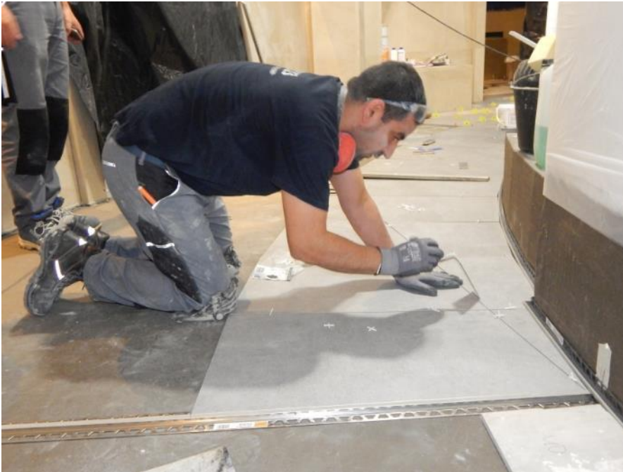
Precision work: due to the special octagonal shape of the room, every single tile was cut to size individually and precisely. ( Link to high-resolution photo, ©PCI Augsburg GmbH)
