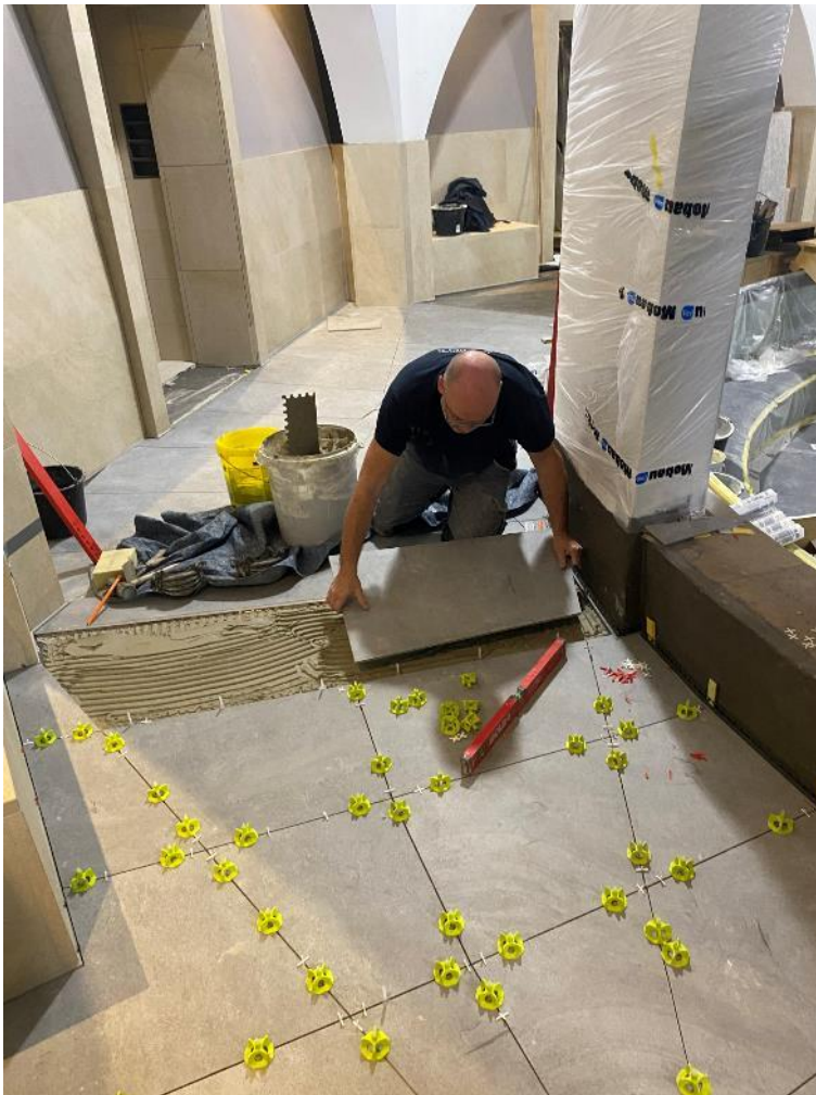
In the relaxation area, the craftspeople laid the large-format tiles with the flexible tile adhesive PCI Flexmörtel S1 Flott which prevents the heavy mega formats from sinking in. ( Link to high-resolution photo, ©PCI Augsburg GmbH)
